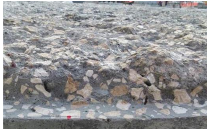
FIGURE 1: CONCRETE SURFACE WITH APPROXIMATELY 50% FRACTURED, COARSE AGGREGATE VISIBLE
