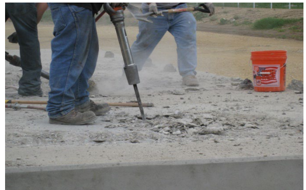
Concrete foundation chipped and abraded
