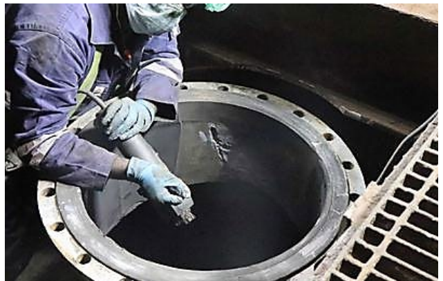
FPF sea water nozzle rubber lining with gouge
