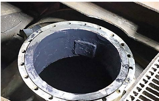
Devcon Flexane General Purpose Putty applied to the repaired surface and on the rubber lining to provide seamless protection
