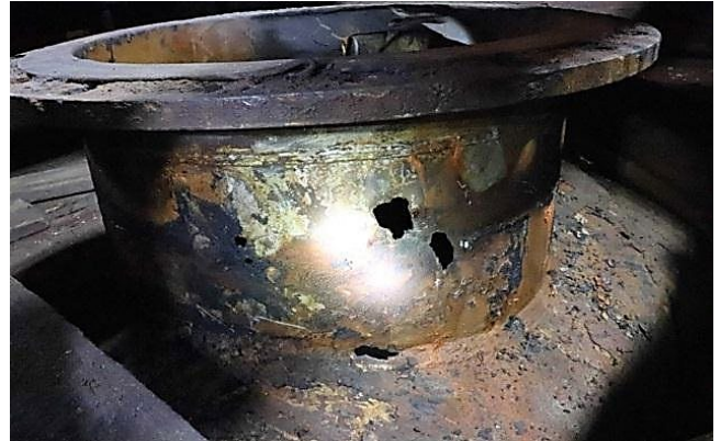
Damaged FPF sea water nozzle (DN600)
