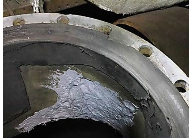
Devcon Plastic Steel 5 Minute Putty (SF) applied to rebuild the missing metal in header interior
