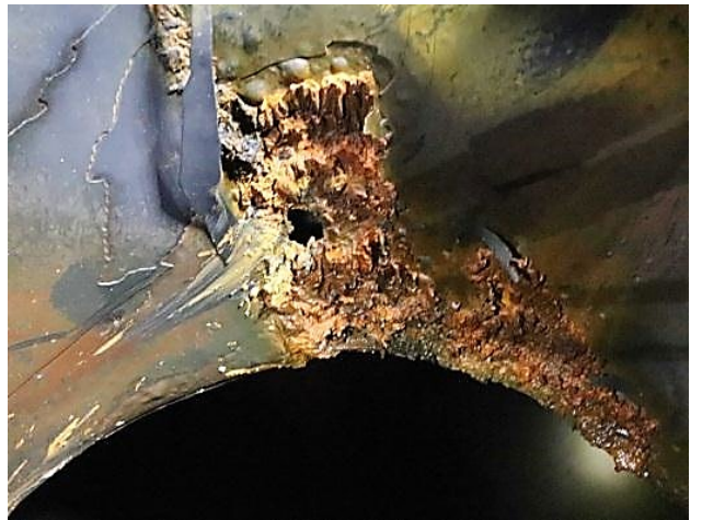
Close-up of corrosion before repair
