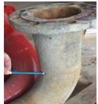
Worn pin hole leaks
