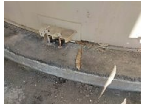
Corroded holding tank
