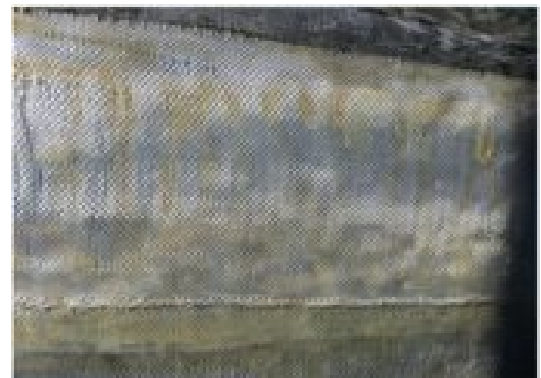
Chemically corroded external tank
