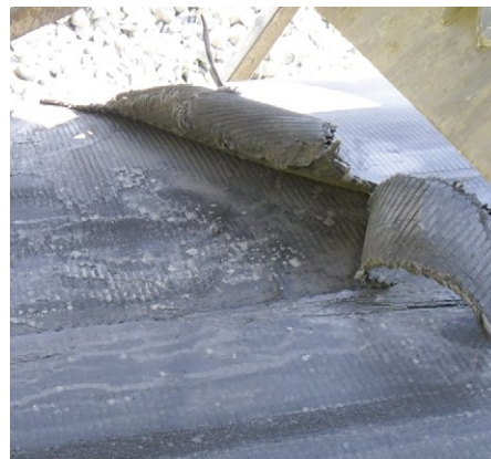
Before Repair: Large tear in belt due to rocks getting caught under the scraper blade.
