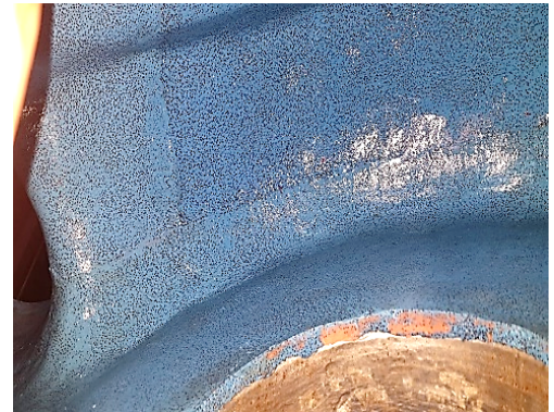
Close up of Devcon Wear Guard 300RTC on slurry pump
