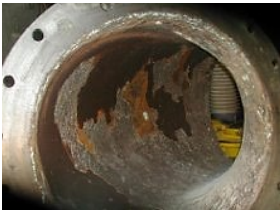
Corroded transfer pipe
