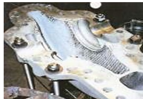
Side view: depicting inside of the corroded fly ash pump
