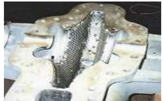
Overhead view: Inside corroded fly ash pump
