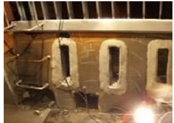
Damaged drain face
