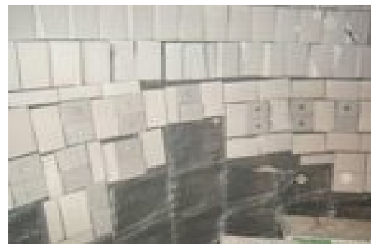
Damaged ceramic tile
