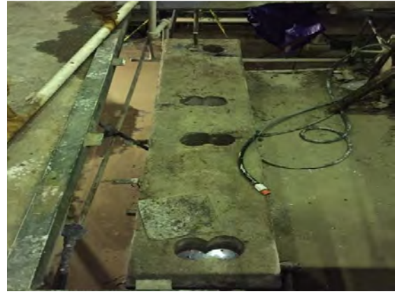
Figure 6: Foundation After Damaged Anchor Bolts Removed
