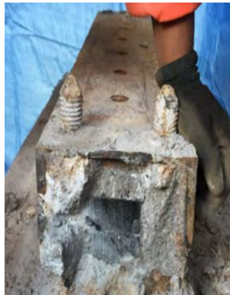
Figure 3: Degradation of Existing Cementious Grout under Support Rails
