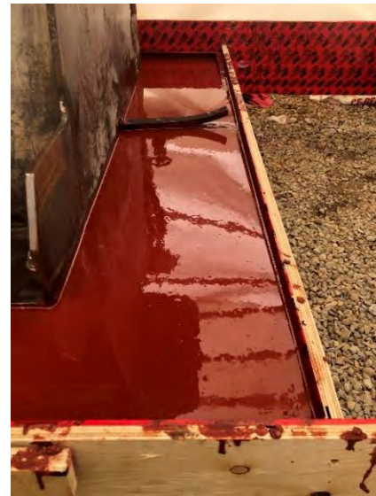
Figure 17: Superior Epoxy Grout Installed in New Anchor Bolt Pockets and Under Baseplate and Baseplate Extension
