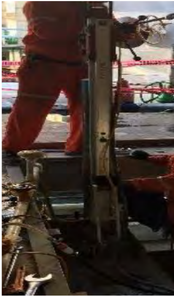
Figure 5: Core Drilling Damaged Anchor Bolts
