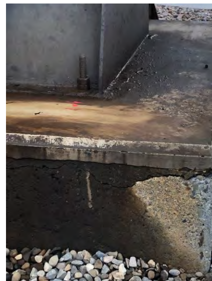
Figure 11: Edge Lifting on Foundation
