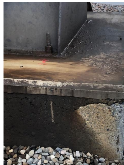
Figure 11: Edge Lifting on Foundation
