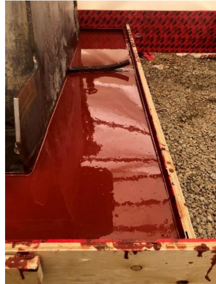
Figure 17: Superior Epoxy Grout Installed in New Anchor Bolt Pockets and Under Baseplate and Baseplate Extension
