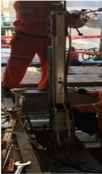
Figure 5: Core Drilling Damaged Anchor Bolts
