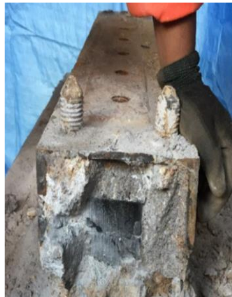
Figure 3: Degradation of Existing Cementitious Grout under Support Rails
