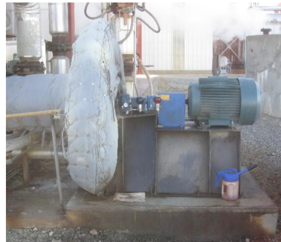
Figure 10: Original Equipment Installation
