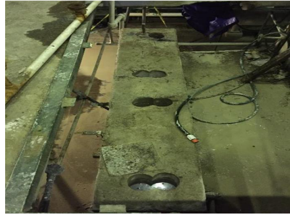
Figure 6: Foundation After Damaged Anchor Bolts Removed
