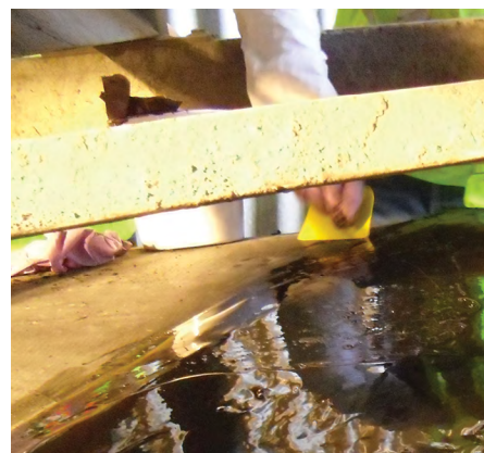
After Repair: Belt flap cut down, Devcon Surface Conditioner and R-Flex applied to belt.
