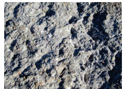
Figure 5: Fractured Coarse Aggregate
